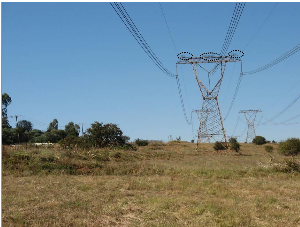
Figure 14: Bird guards (‘spikes’) fitted to a self-supporting tower.
