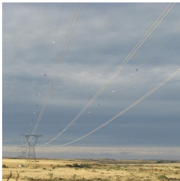
Figure 16: An example of the Double Loop Bird Flight Diverter fitted to the earth wires of a 500 kV transmission line (image courtesy and copyright of Shaw, 2013).
